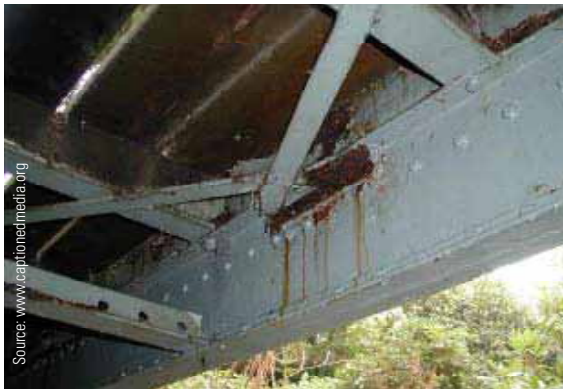
Figure 5.1: Example of corrosion caused by electrolysis
