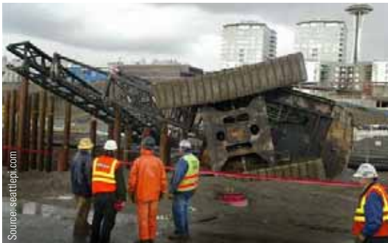
Figure 5.2: Example of crane overbalancing into the rail corridor
