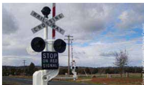
Figure 5.4: 'Active protection' at a level crossing
