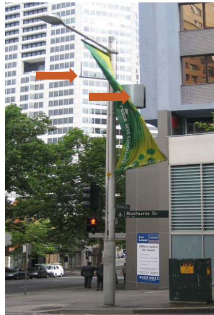
A microcell omnidirectional antenna attached to an existing street light pole (extending to the left under the light) and accompanying equipment unit (attached to the right).
