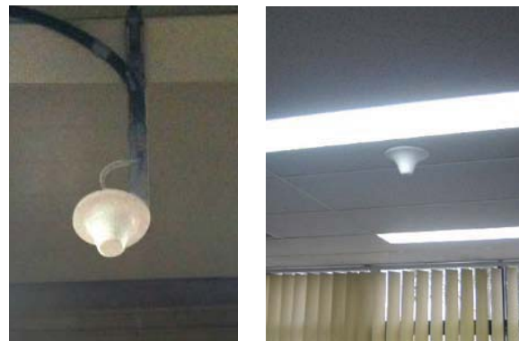
Left-right: Picocell antenna suspended from a ceiling; A cone shaped picocell on a ceiling.
