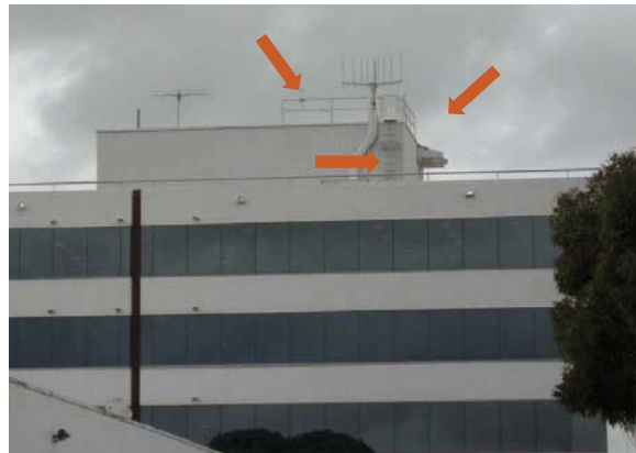
Rooftop installation with colour matched cable tray, safety rail and ladder
