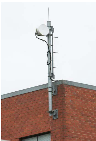
A radiocommunication dish used to send a radiofrequency signal from a macrocell base station to another base station (line-of-sight).
