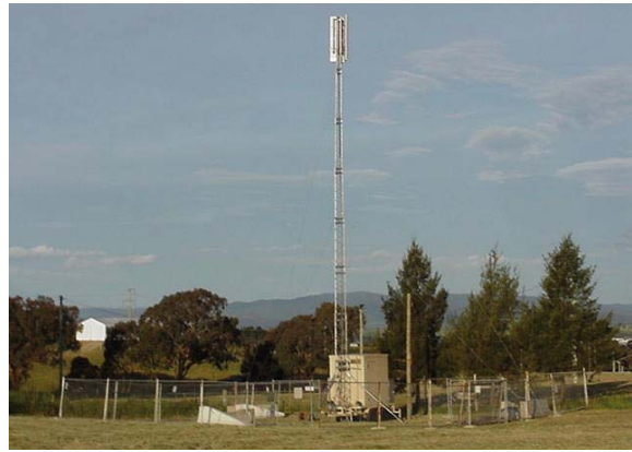
Temporary macrocell base station (consisting of two panel antennas) on lattice support mount deployed at a sporting event.
