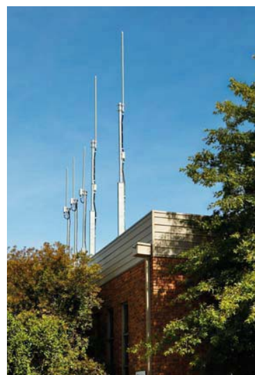
An array of omnidirectional antennas.
