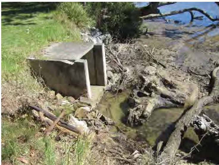
Figure 39: Stormwater outlet at Mossy Point causing scour of bank
