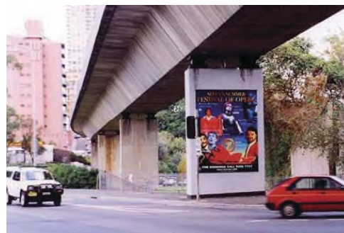
✓ ADVERTISEMENT WITHIN STRUCTURAL BOUNDARIES OF RAIL BRIDGE
