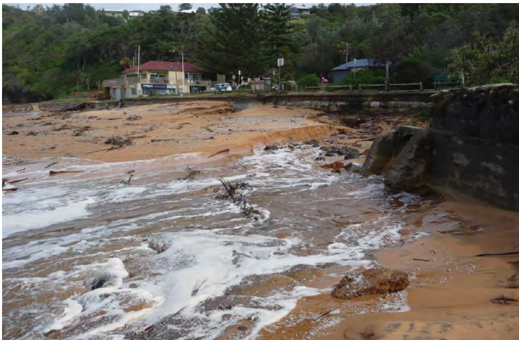
Figure 20: View of scour at northern end of Bilgola SLSC seawall and adjacent to Bilgola Creek and Bilgola Kiosk channel
