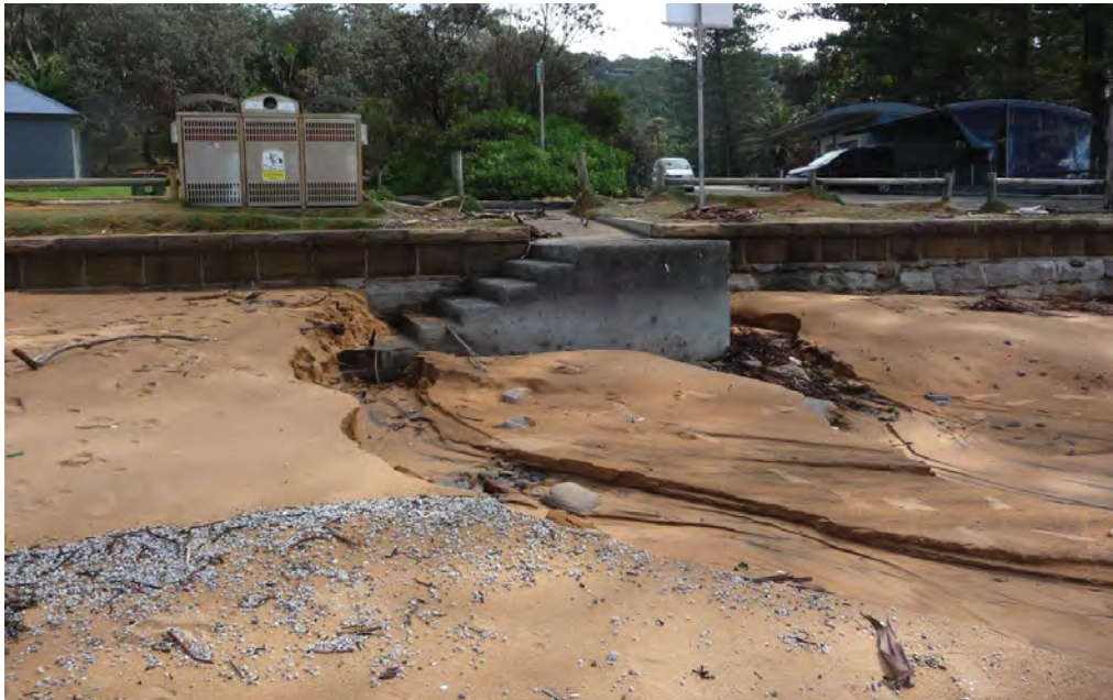
Figure 19: Scour at Bilgola Beach car park seawall steps
