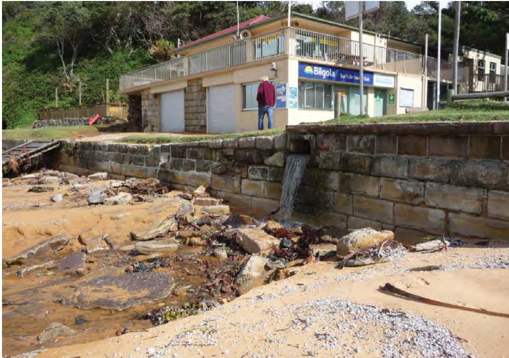
Figure 21: Scour at Bilgola SLSC stormwater outlets
