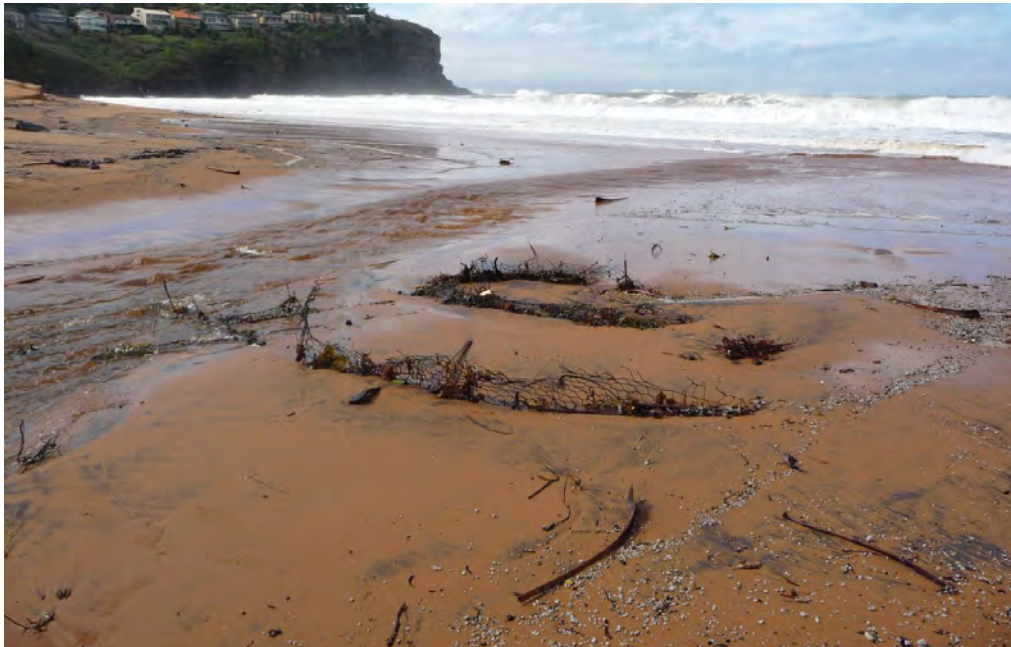
Figure 15: Deteriorating wire from gabion basket or reno mattress scour protection seaward of Bilgola Creek
