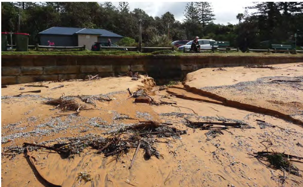
Figure 18: Scour at southern shower at Bilgola Beach car park
