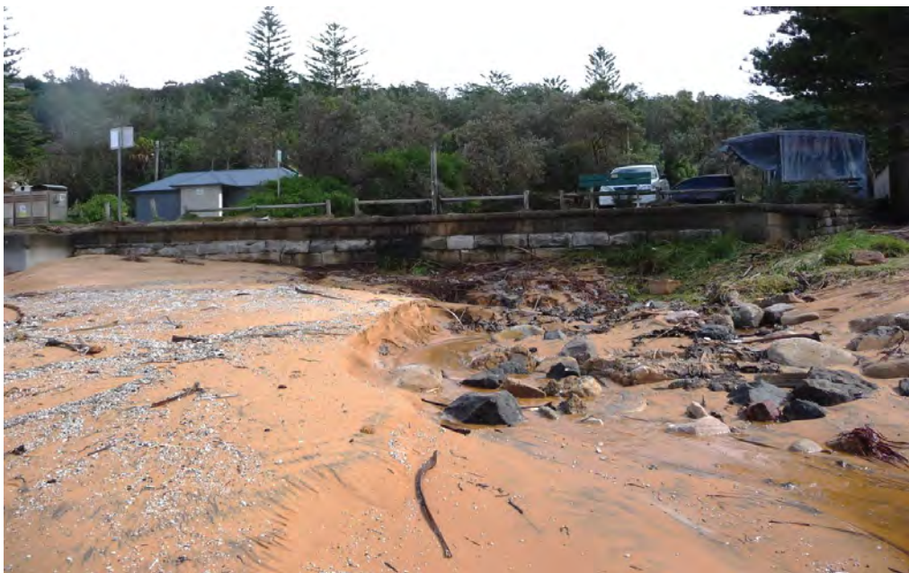
Figure 16: Rocks exposed seaward of Bilgola Kiosk channel outlet
